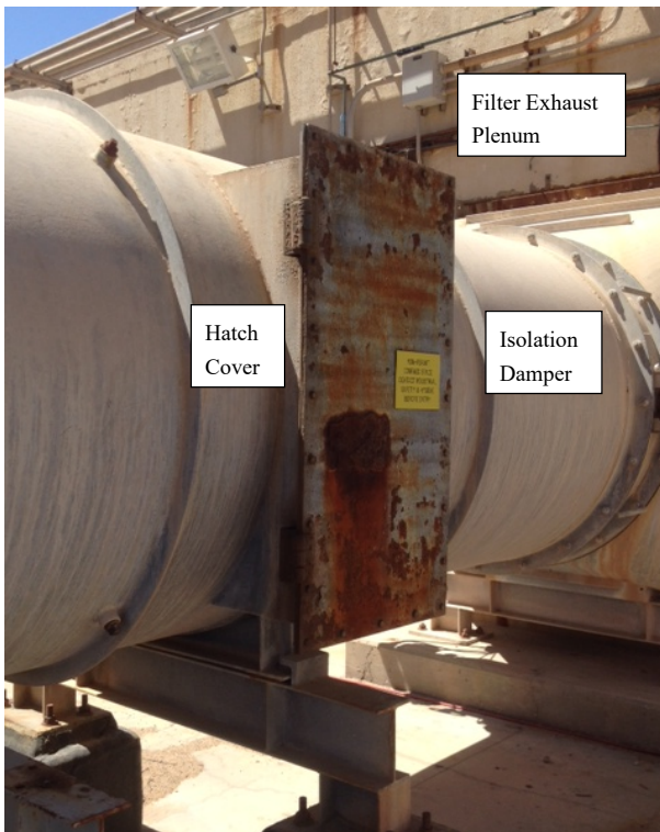
Fig. 8. 860 fan access hatch with isolation damper.
